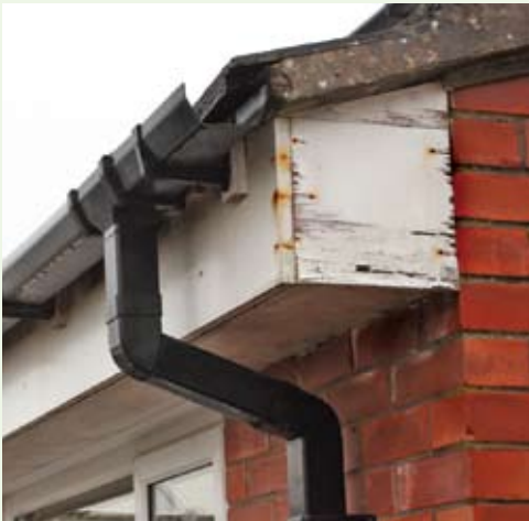
Timber roofline can rot without maintenance...
