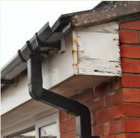
Timber roofline can rot without maintenance...
